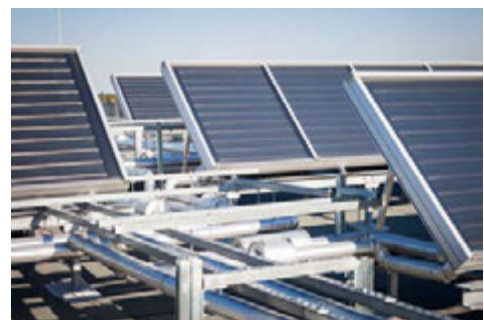
Solarpanele | © Adam Sevens
